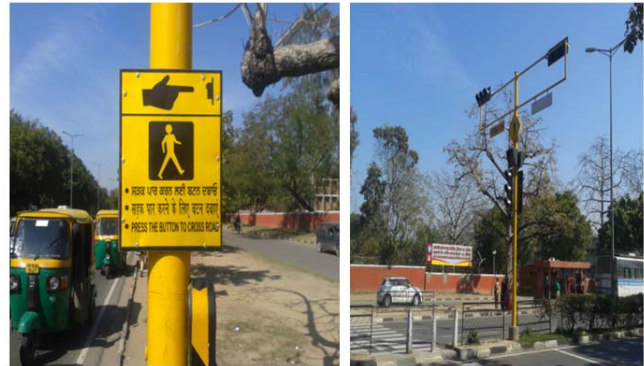
Fig. 1: Installed PELICAN Signal at Madhya Marg Chandigarh
